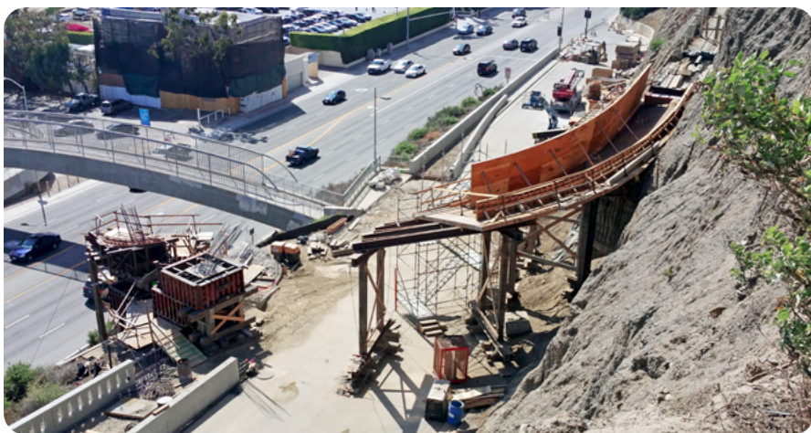
Construction of the Idaho Trail pedestrian overcrossing on May 27, 2016. Photo by Gary Bonart.
