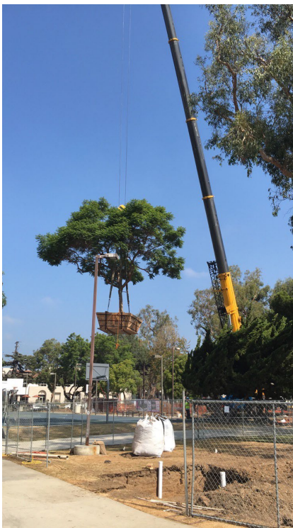
Onsite Jacaranda relocation as part of Reed Park landscape improvement & exercise area retrofit.
